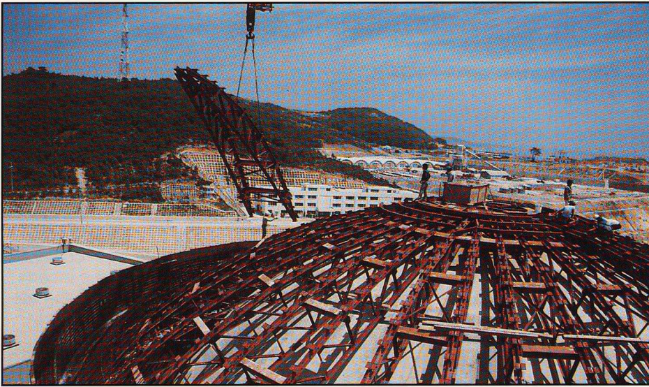
Westinghouse constructed Korea's KOR1 2 on a nuclear island turnkey basis. The plant was built within a 63-month schedule.
